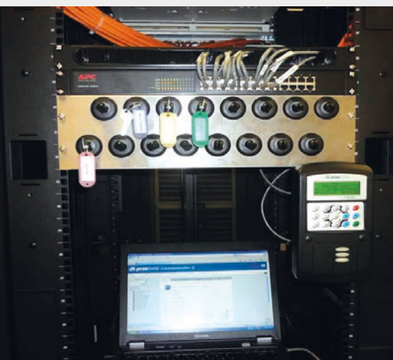
Key panels can be easily mounted on server racks.
